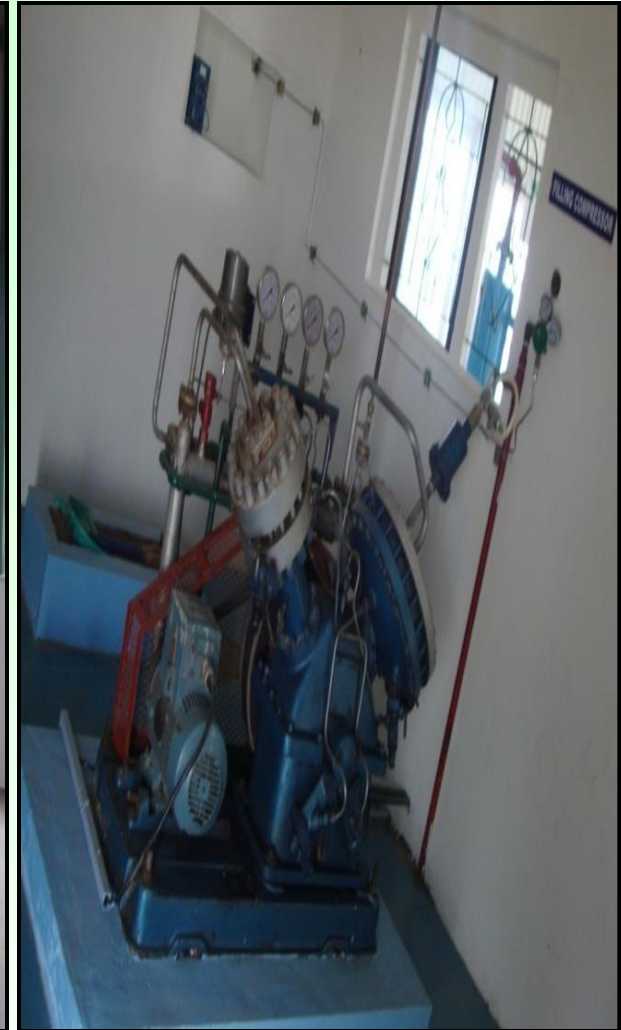
High Pressure Compressor at Nasik plant
