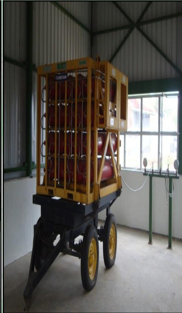
Cylinder Cascade for bottled biogas
