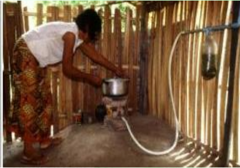
Pipeline for raw biogas use as a cooking fuel
