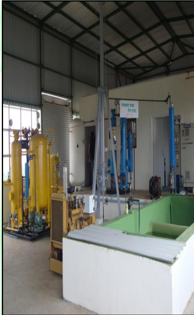
Water Scrubbing and PSA system at Nasik
