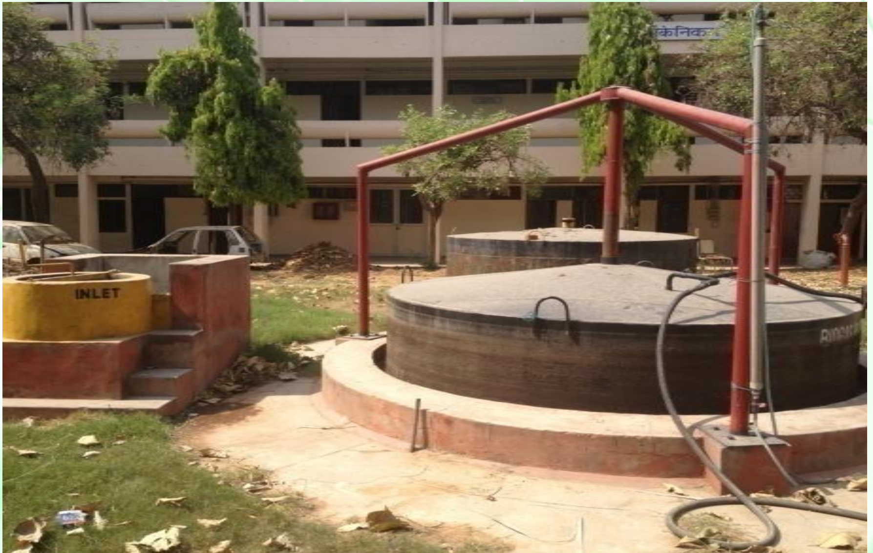
Biogas Plant at IIT Delhi
