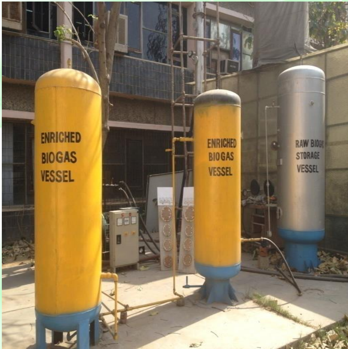
Raw and upgraded biogas storage vessels
