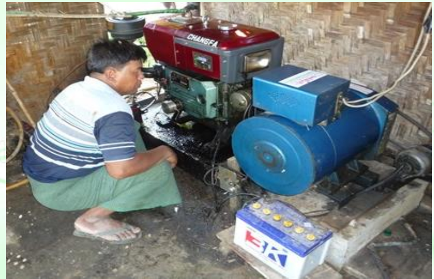
Biogas Engine for electricity production
