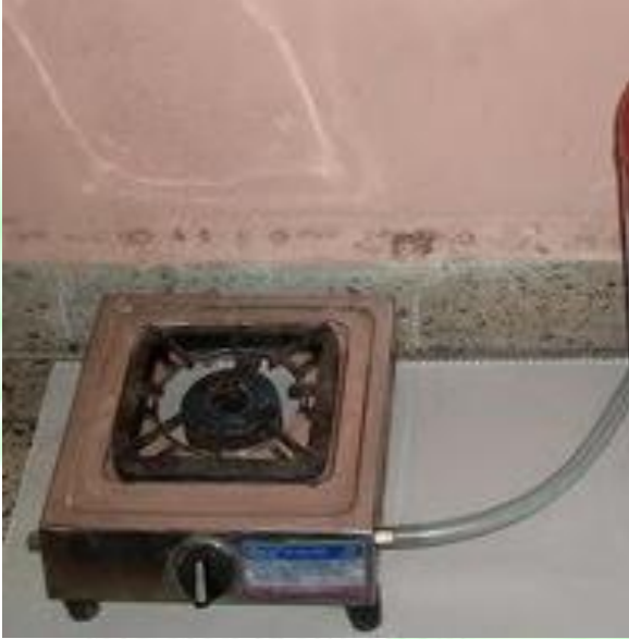
Upgraded and bottled biogas for use as a cooking fuel
