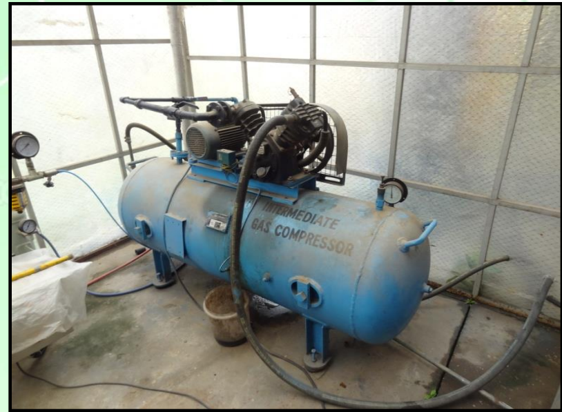
Intermediate Gas Compressor
